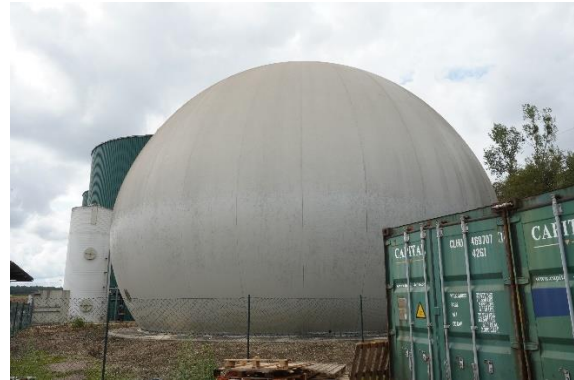
Biogas storage 2500m 3 . The CHP produces 1600 kWh. All of the process heat is used in the plant itself.
