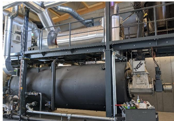
Pyrolysis plant. The heat from the process is cooled down to 300°C and used for drying sewage sludge.
