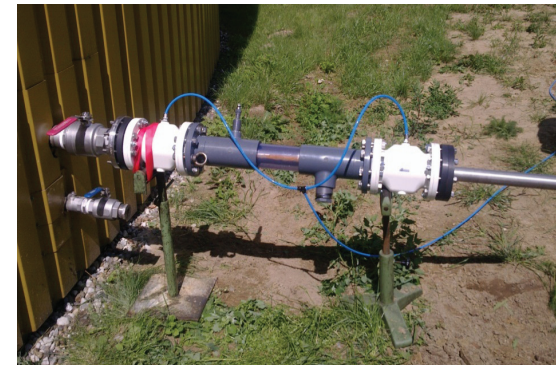
Figure 50: Example of a lock chamber for rinsing and sealing of the sensor (Source: TU Berlin)
