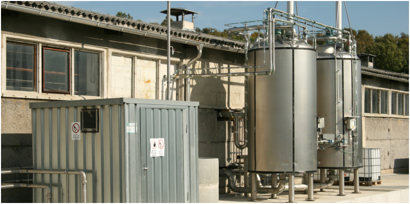
Figure 7.3-3: Pilot biogas plant Fraunhofer IKTS
