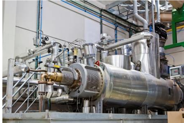
Figure 5. Torrefaction reactor in CENER facilities
