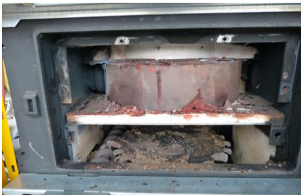
Slag deposits (underfeed boiler)
