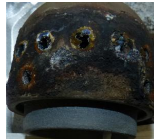
Air nozzles clogged, (overfeed boiler)
