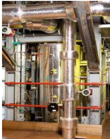
Torrefaction Section of the reactor
