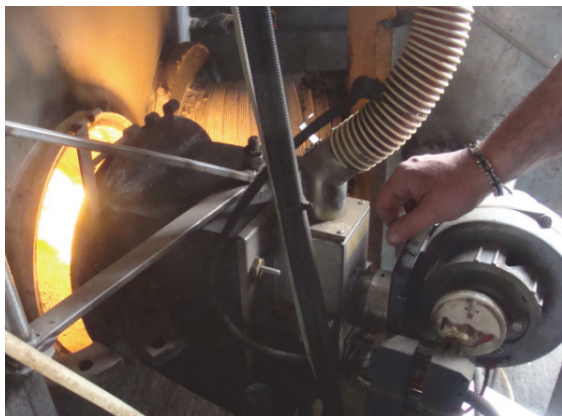
The pellet burner of 60 kW.
