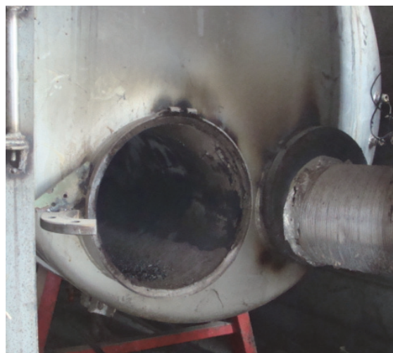
Boiler in the dairy of Mr. Tommasoni.
